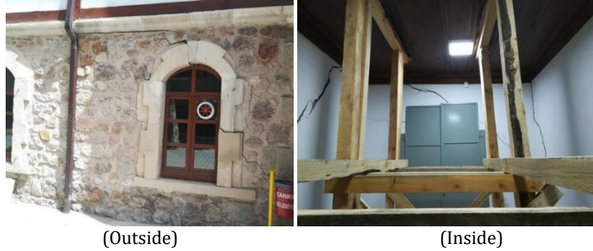
Figure 15. Cracks seen on the walls in 2019 (Ankara Directorate for Surveying and Monuments, 2021).
