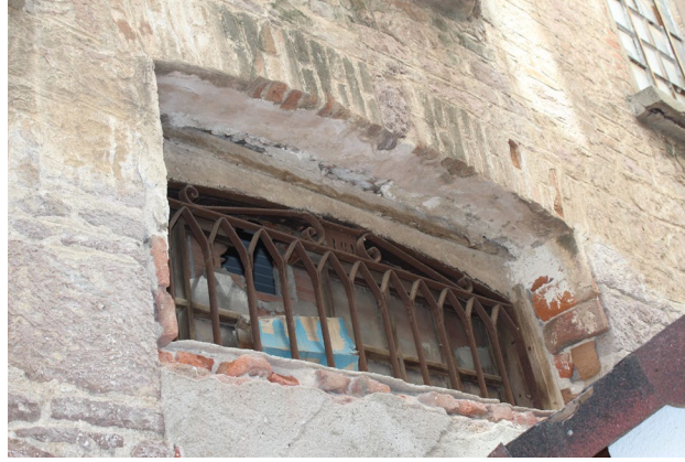
Fig. 9. "1911" Written Plate on the Iron Bars of the Window on the North Façade (Photographed by Interior Architect Elif Türkmen)
