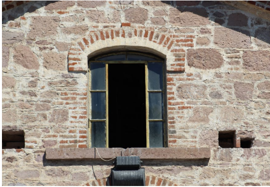
Fig. 15. Skylight Window on the Upper Level of the First Floor, Proving the Presence of an Attic (Photographed by Interior Architect Elif Türkmen)
