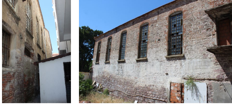
Fig. 20. South/Rear and Lateral Facade of the Soap Factory Building Photographed by Interior Architect Elif Türkmen
