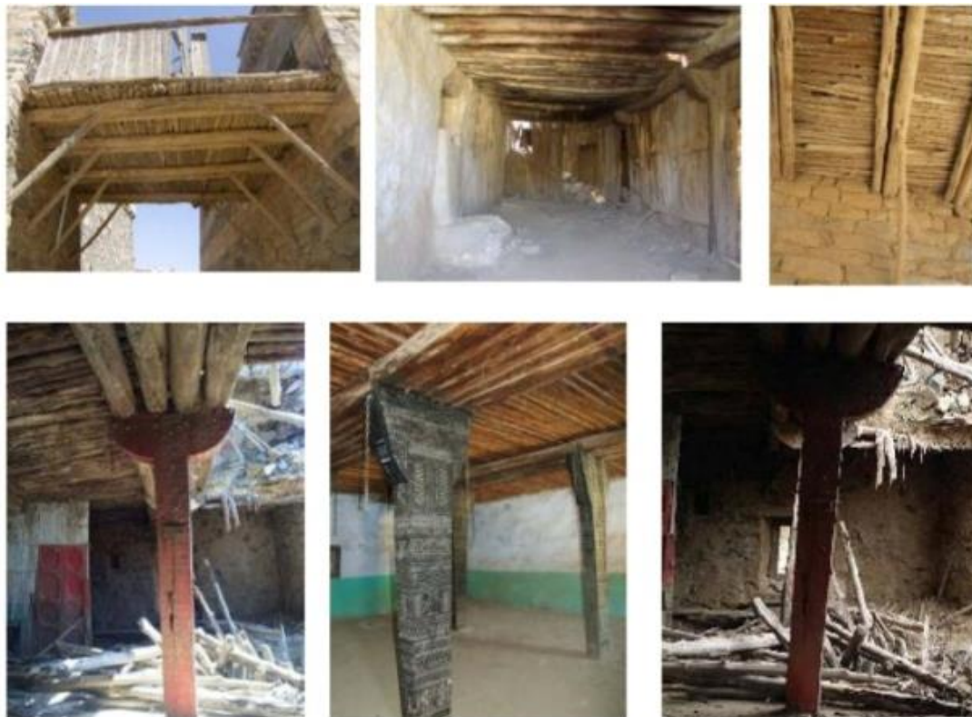
Figure 7. Logs of trees called "Zafer", are used as pillars to hold the ceilings while the veins of trees were used as beams (2018)
