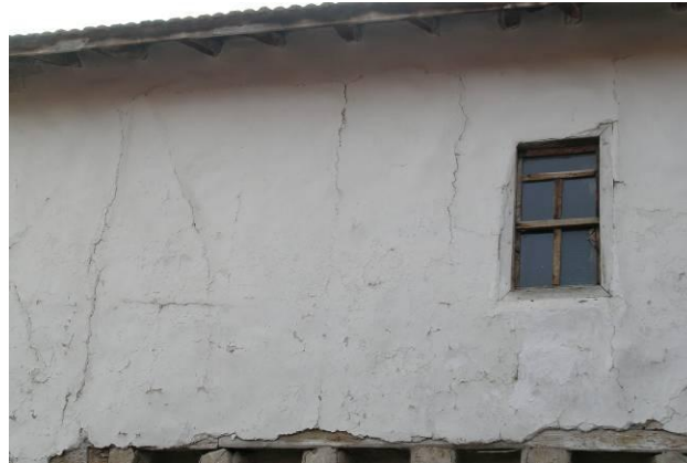
Figure 5. Cracks in a timber-framed structure.
