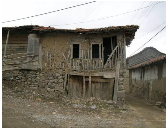
Figure 8. Composite structure: Stone masonry first floor and timber-frame with stone infill (Ortabayındır Village).
