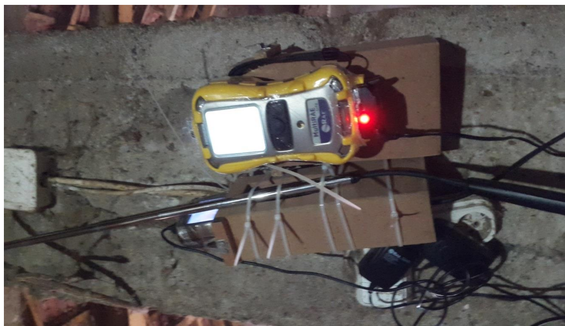
Figure 2- The general condition of measuring devices in the shelter
