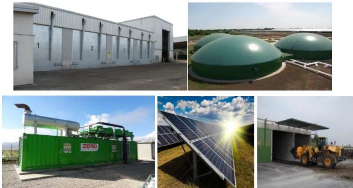
Figure 4. The main elements of the hybrid energy plant.
